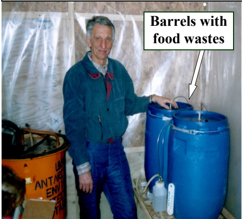
The industrial plant for digestion of solid food wastes at Antarctic station
